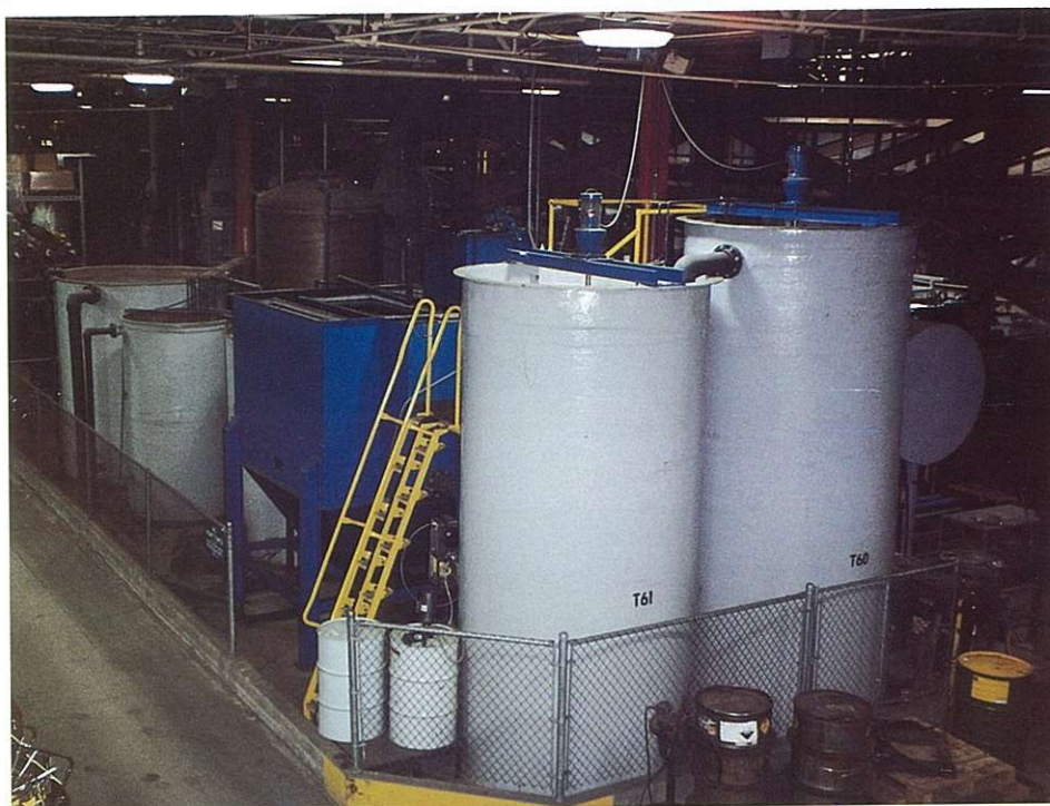
120 GPM turn key installation on nickel/chrome plating waste.
