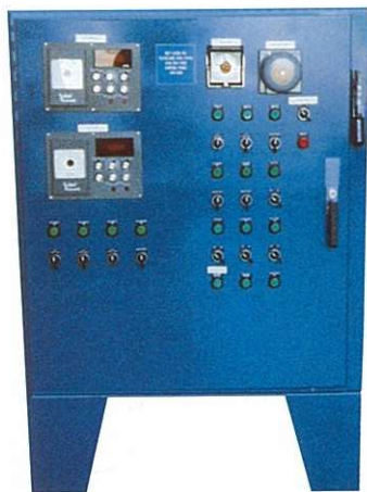
Custom built control panel for 60 GPM system on zinc phosphate waste.
