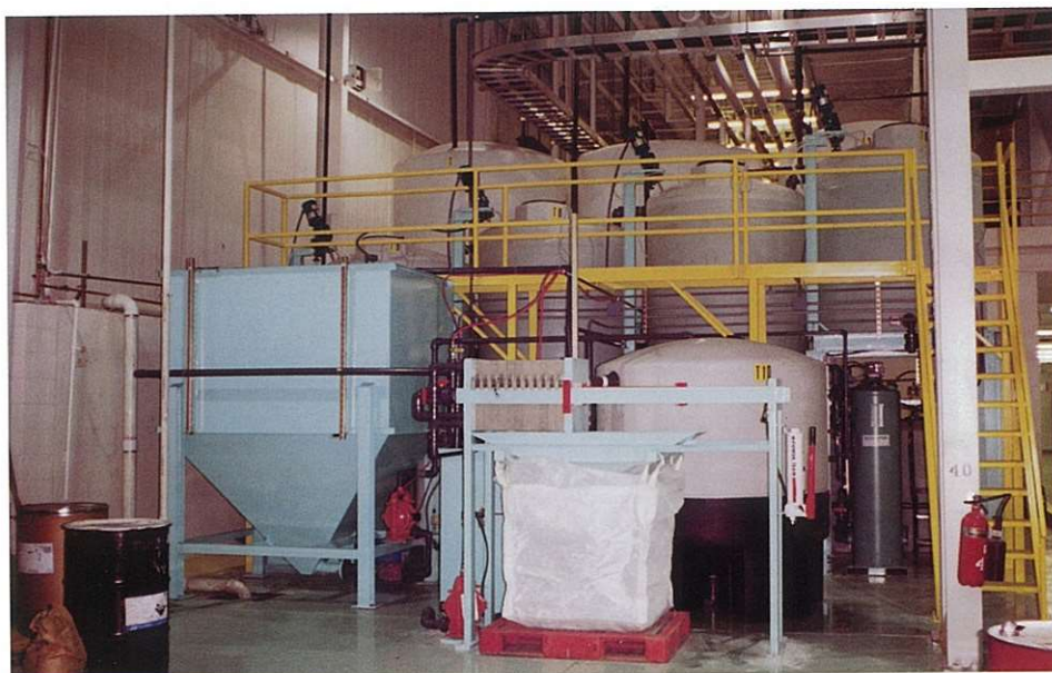
30 GPM system for cyanide and chrome waste water with end of pipe multi-media and carbon filters for water recycle.
